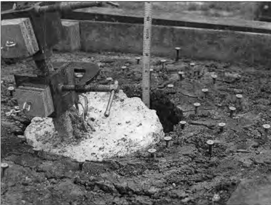
Figure 166 – Gap in Front of Pile (115-mm Pile in Glacial Till)
